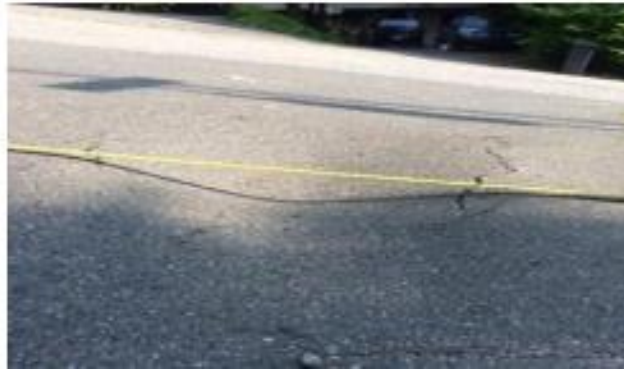
Gambar 3.7 Amblas ( Depression ) Sumber : Bina Marga No. 03/MN/B/1983
