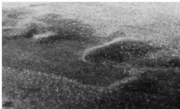
Gambar 3.8 Sungkur ( Shoving ) Sumber : Bina Marga No. 03/MN/B/1983
