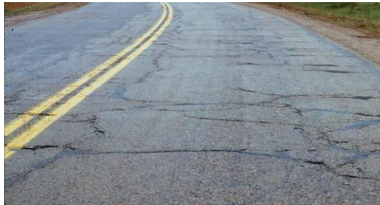
Gambar 3.16 Retak Blok ( Block cracks ) Sumber : Bina Marga No.03/MN/B/1983
