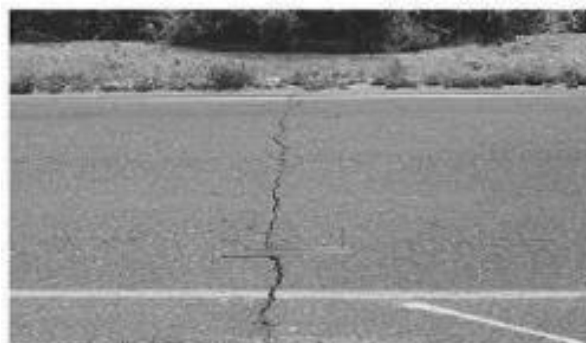
Gambar 3.13 Retak Melintang ( Transverse Cracks ) Sumber : Bina Marga No.03/MN/B/1983
