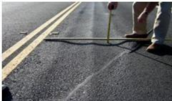
Gambar 3.6 Alur ( Rutting ) Sumber : Bina Marga No.03/MN/B/1983
