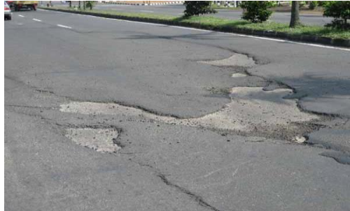
Gambar 3.23 Pengelupasan ( Delemination ) Sumber : Bina Marga No.03/MN/B/1983
