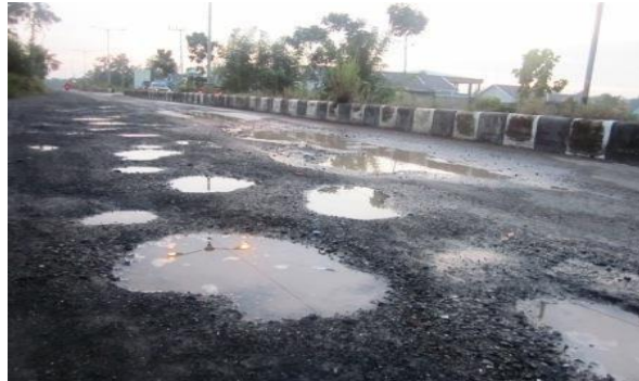
Gambar 3.25 Lubang ( Potholes ) Sumber : Bina Marga No.03/MN/B/1983
