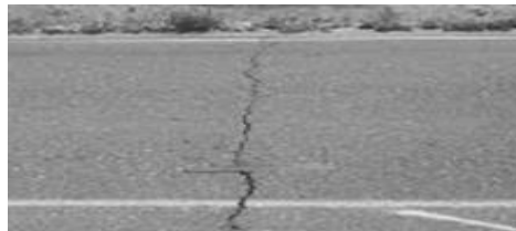
Gambar 3. 14 Retak Melintang ( Transverse Cracks )
