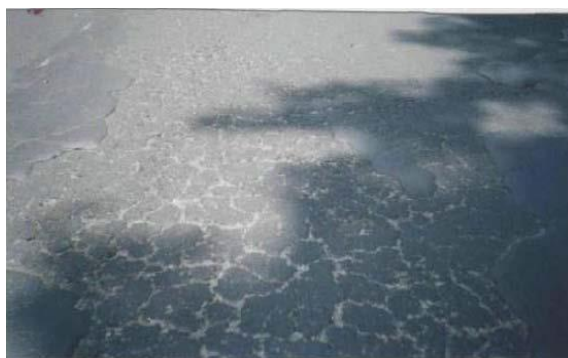
Gambar 3. 20. Pelepasan Butir ( Weathering/Raveling ) Sumber : Bina marga no.03/MN/B/1983
