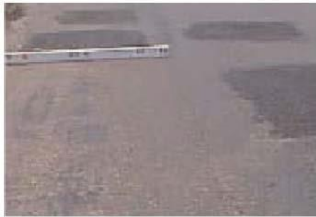
Gambar 3. 12. Tambalan ( Patching end Utiliti Cut Patching ) Sumber : Bina marga no.03/MN/B/1983
