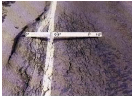
Gambar 3. 17. Sungkur ( Shoving ) Sumber : Bina marga no.03/MN/B/1983
