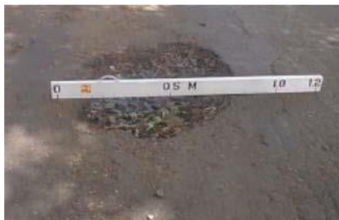
Gambar 3. 14. Lubang ( Pothole ) Sumber : Bina marga no.03/MN/B/1983
