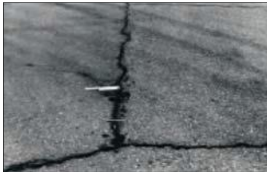
Gambar 3. 9. Retak Sambung ( Joint Reflec Cracking ) Sumber : Bina marga no.03/MN/B/1983
