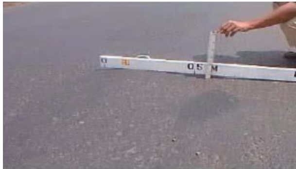
Gambar 3. 16. Alur ( Rutting ) Sumber : Bina marga no.03/MN/B/1983
