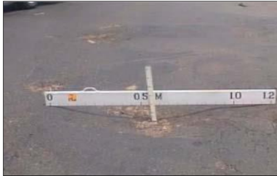
Gambar 3. 7. Amblas ( Depression ) Sumber : Bina marga no.03/MN/B/1983
